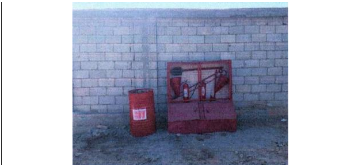
Figure 17. Firefighting equipment at TSS Hakkulabad
