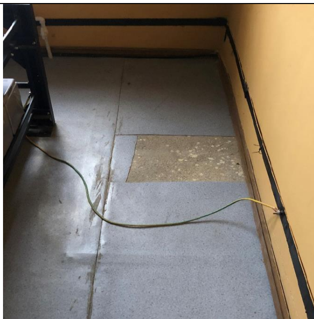
Figure 6. Grounding of floor devices at Namangan station does not comply with the standards (2022).
