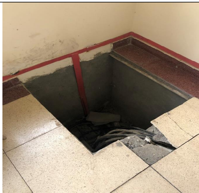
Figure 7. There is no floor covering, which leads to a violation of the safety of personnel at the Namangan station (2022).
