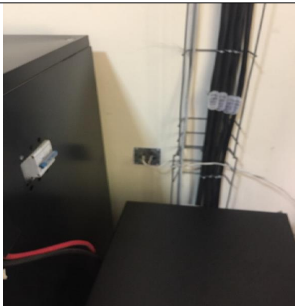
Figure 5. Violation of fire safety rules at the Uychi station (2022).
